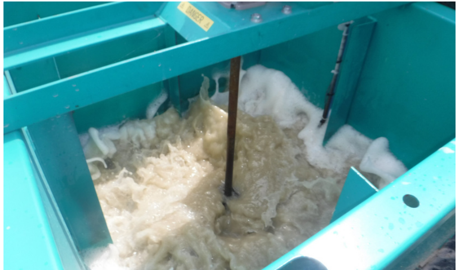
EnviroHub TT01 Concrete Water Treatment Unit neutralising the alkaline pH levels of the wash water for reuse or safe disposal.
