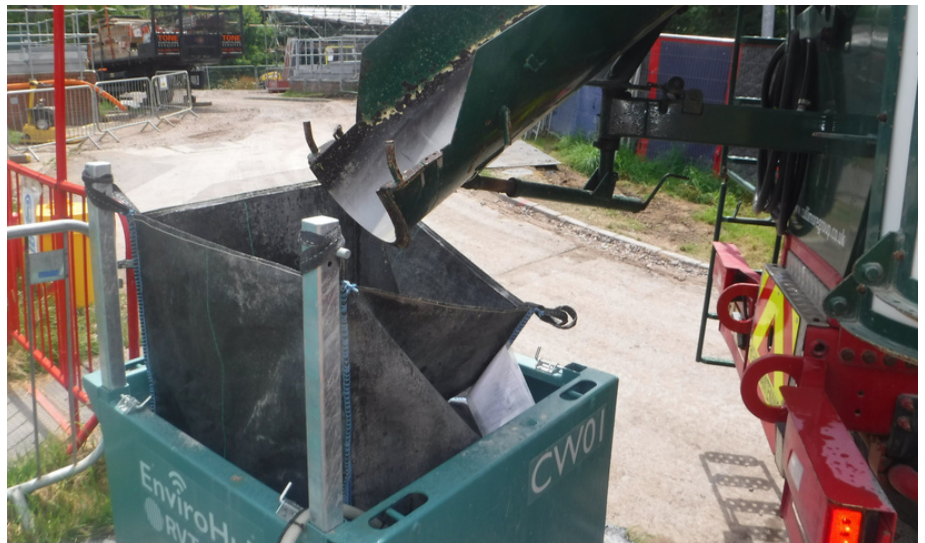
EnviroHub CW01 Concrete Washout Unit and geotextile filter bag separating the solids from the wash water.
