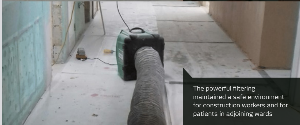
Powered by 110v droppers to minimise cabling on the floor
