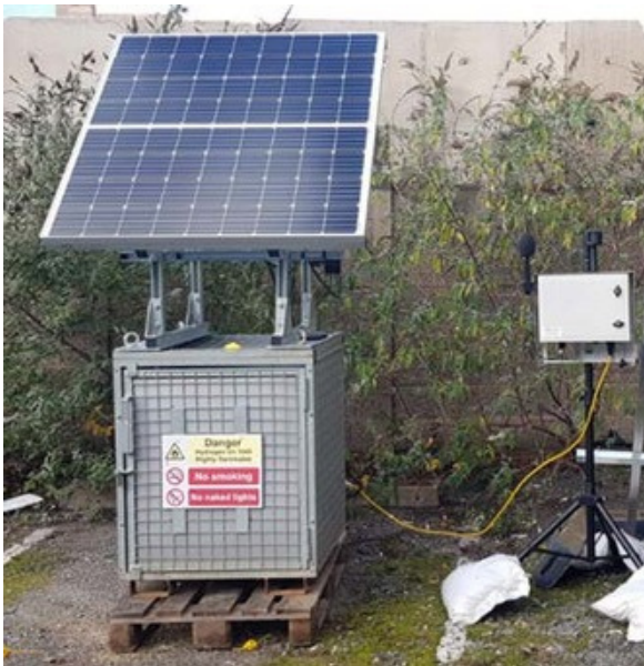
Eco-CH 2 Cabinet and Cage in use with RVT's MONITEX Noise Monitor
