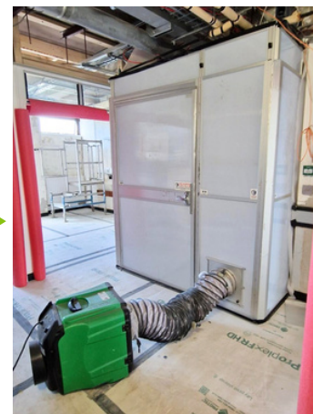
The DUSTEX® Raptor is creating positive pressure inside the containment unit, so that if the door is opened, it will push the air back into the respective area.
