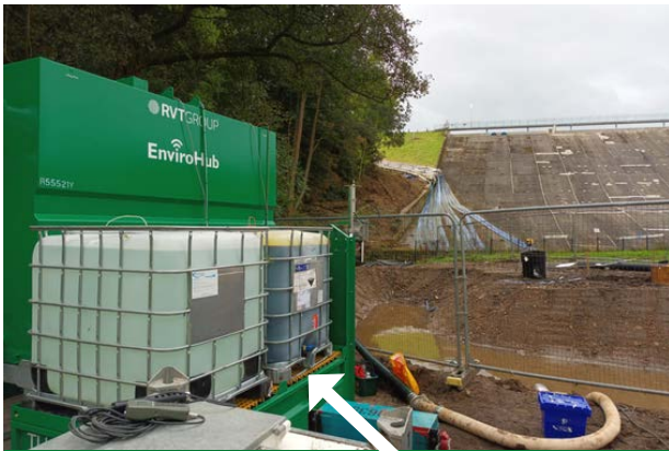
The EnviroHub TU02 Dosing Skid is used with water treatment tanks to automatically add flocculant and coagulant
