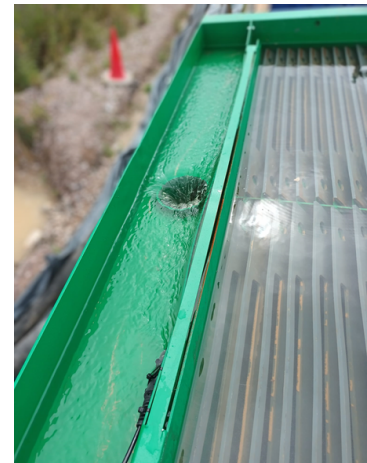
The water settlement tank is a simple but effective way of separating solids from water on site.
