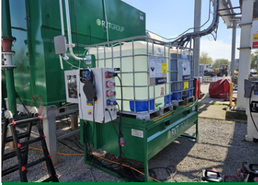
EnviroHub® TU02 Dosing Skid adding chemicals to the Treatment Tank.
