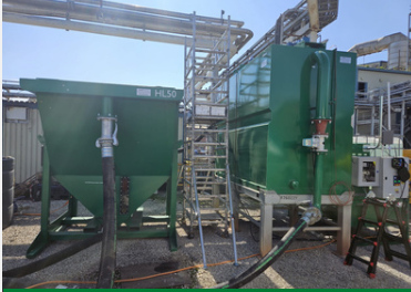
EnviroHub® TT10 Treatment Tank (right) and HL50 Lamella Settlement Tank (left).
