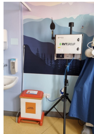
RVT's Noise Monitor inside a children's ward, continuously monitoring noise pollution.
